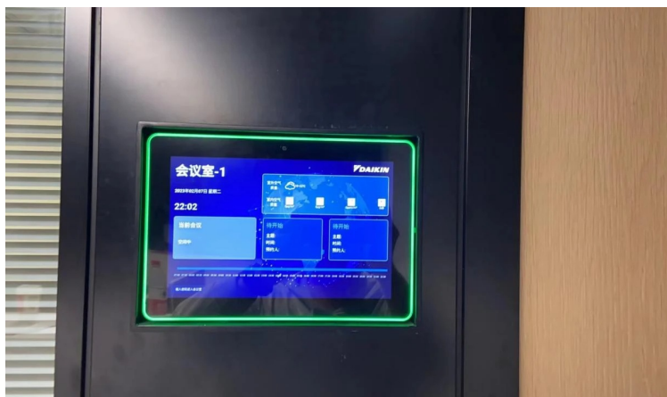
Daikin Guangzhou smart office
