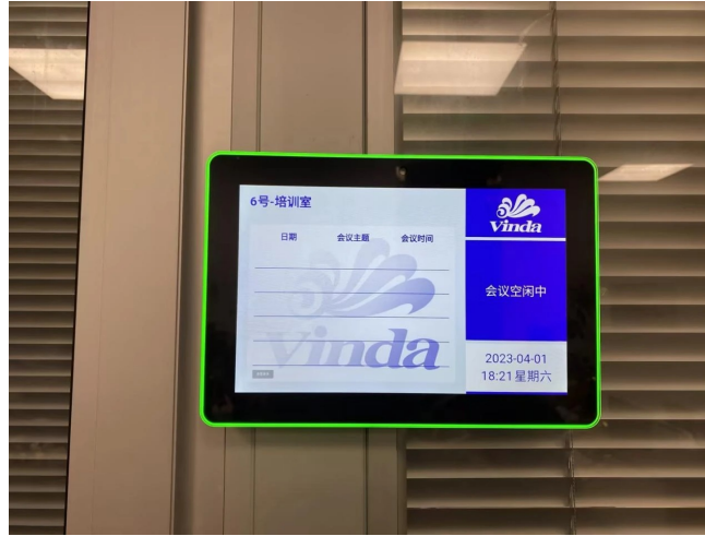
Vinda Guangzhou smart meeting project
